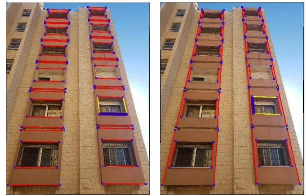
a) b) Figure 9. Image lines: a – image lines for horizontal object lines; b – image lines for vertical object lines
