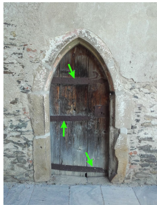
Figure 14. Wösendorf – Romanesque wrought iron door hinges (marked by the arrows) are fixing the boards of the door
