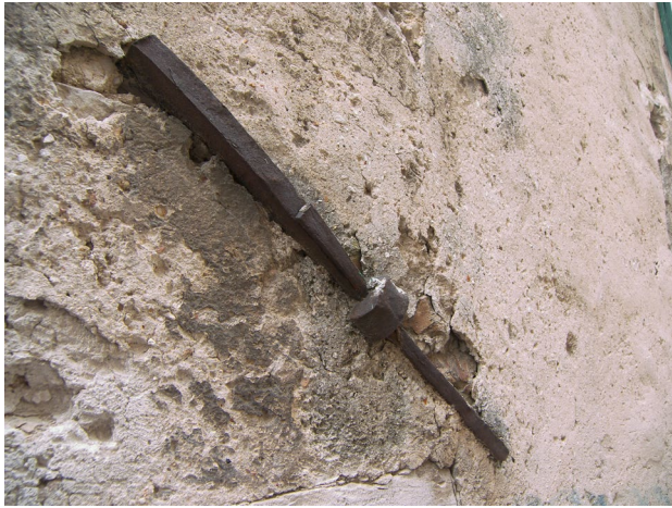
Figure 4. Sibenik – undecorated wrought iron ties – originally placed under the plastered surface
