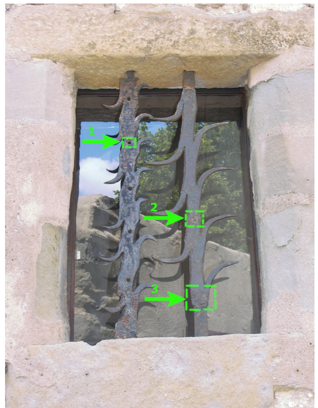
Figure 20. Carcassonne, Window grill made of different wrought iron straps – punched holes (arrow 1) and rivets (arrow 2) without present function, and subsequent welding (arrow 3) give evidence of the secondary use
