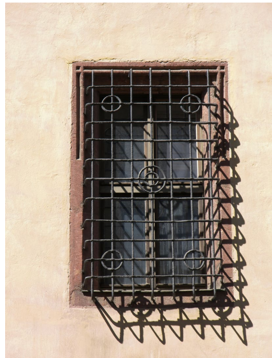
Figure 12. Leipzig – typical wrought iron window grill: the composition of bars is the optimal utilization of the fibrous material, that makes easier lengthening (longitudinal transformation) than widening (transversal transformation)
